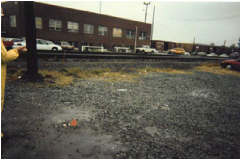
Photograph 3 After treatment the injection points were left in place but cut off at ground level.
